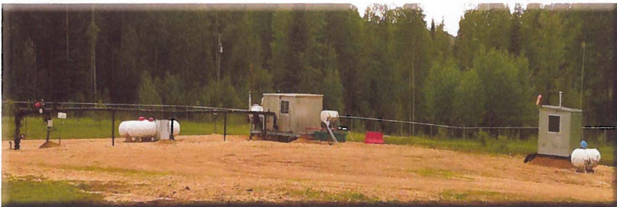
Natural gas facility
