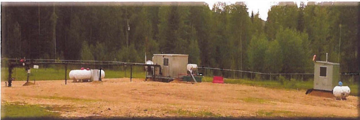
Natural gas facility
